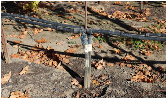
Figure 6 Properly installed irrigation gate valve, fertilizer injection port at the correct height of 55 cm above vineyard floor.
